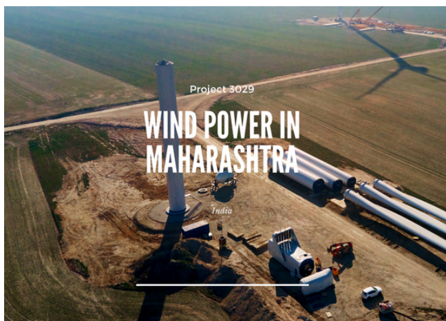
Project 3029: Wind Power in Maharashtra
